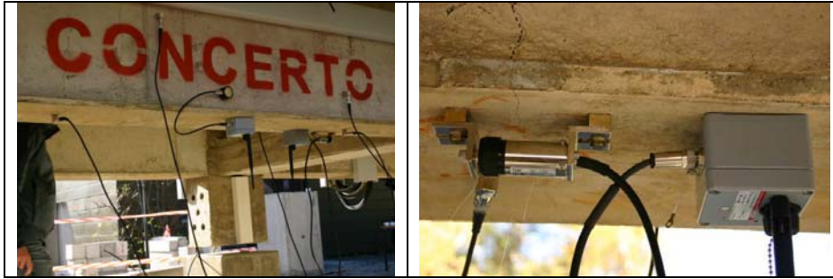
Fig. 4: “Concerto Bridge” in Brunswick equipped with wireless AE sensors (left) and with wireless strain sensors (right)
