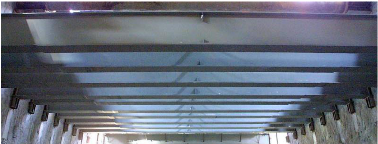
Figure 2: Photo of as-built soldier-pile tremie-concrete slurry wall and composite steel-and-concrete roof system
